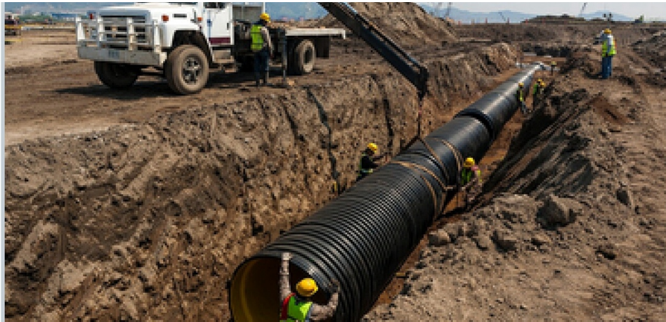
Figure 4.2. Climate resilience is also a pipe problem: water, wastewater, reuse, and industrial fluids must move through systems that waste less.
